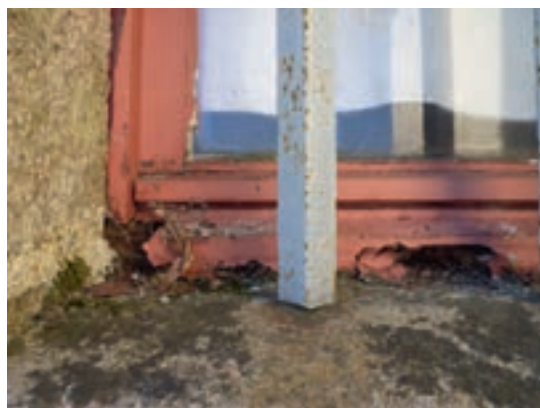
▲ Menuiseries moussues, bois altéré
